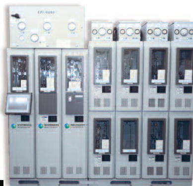
Point of use purification to assure process consistency.
