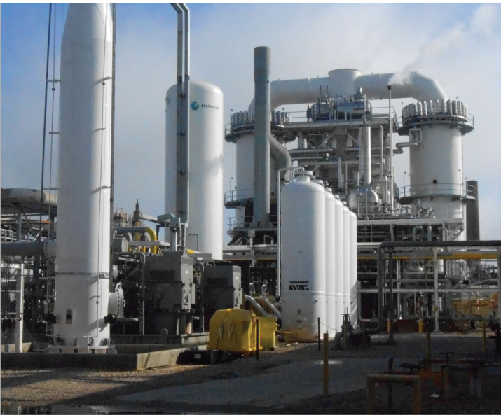
Nippon Sanso Matheson Steam Methane Reformer, Pensacola, FL
