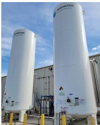
Bulk tanks with Trifecta® Supply System
