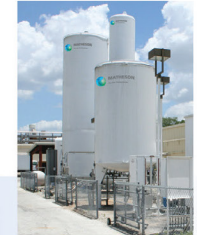
Onsite Plants and Pipeline
