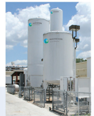
Onsite Plants and Pipeline
